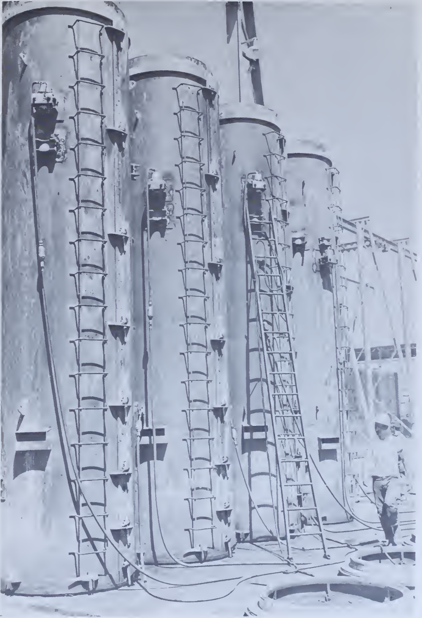
Figure 160.—Casting 20-foot lengths of 54-inch-diameter pipe. The concrete is consolidated by two form vibrators per pipe. PX-D-33052.
